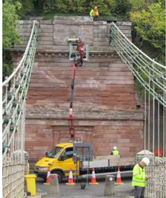
Surveyors check the masonry on the English tower during the current Bridge closure; 21 st September
